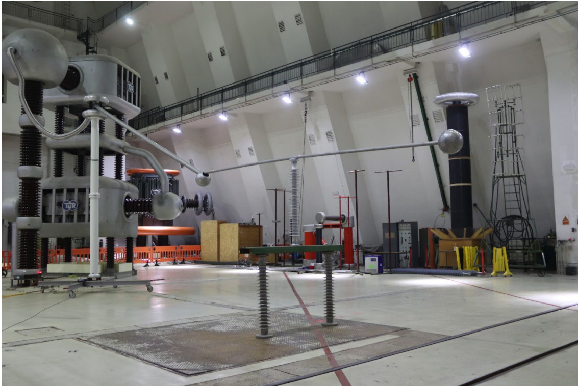
Figure 3 Test arrangement during the radio-influence voltage test
